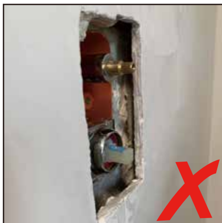
Valve installed too deep- incorrect installation
