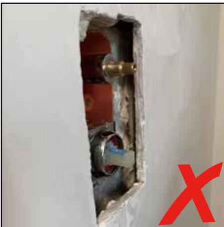
Valve installed too deep- incorrect installation
